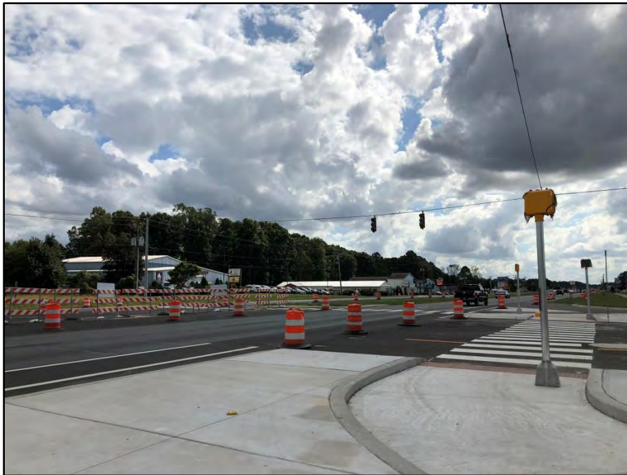
Newly constructed traffic signals at the future intersection of Route 13 and the Camden Bypass
